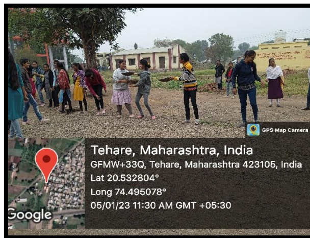
NSS Volunteers repairing the road and cleaning area near Tehere Grampanchayat Office
